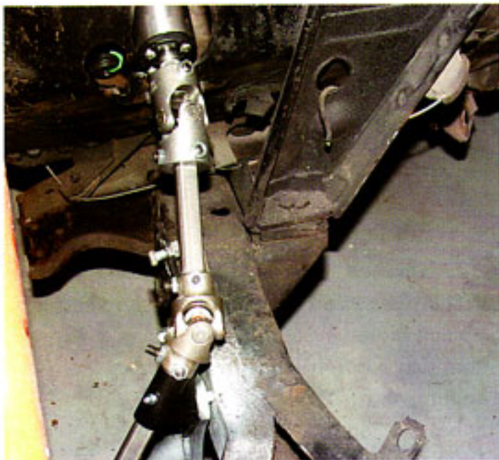
Photo #8: With the upper shaft cut to length, install the shaft into the upper U-joint and center U-joint and lock into place with the set screws.
